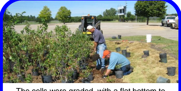
The cells were graded with a flat bottom to spread the stormwater flow more evenly. Native shrubs, wood mulch and perimeter sod were installed.
