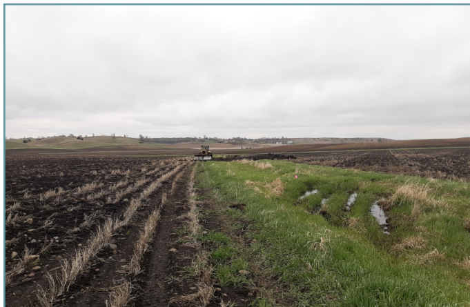
Prior to construction, sediment build up was causing saturation and out of bank flow due to lack of capacity.
