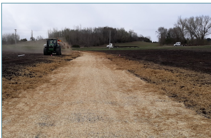
Erosion control blanket and mulch were installed to reduce erosion until vegetation is fully established.
