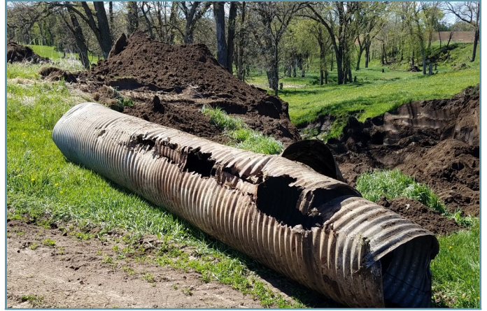
The pipe had rusted through and needed to be removed.
