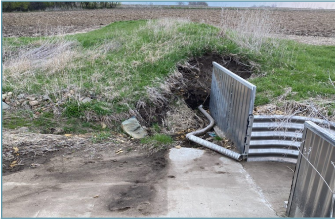
High flows had eroded around the end of the existing wing wall and scoured alongside the existing concrete slab.
