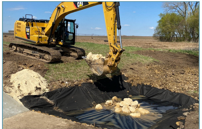
Rock riprap was installed over geotextile fabric to prevent scour at the end of the concrete slab.
