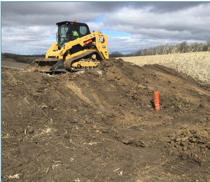
Embankment was repaired by compacting soil and grading to match the original design.
