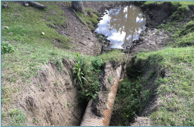
The existing pipe, originally installed in 1958, was no longer functioning and erosion had occurred alongside the pipe.
