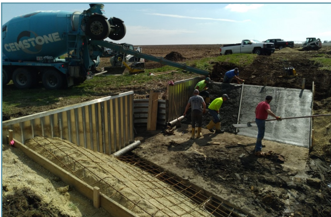
Concrete pads were installed on both sides of the existing concrete slab
