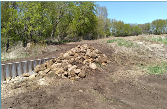
Riprap was placed to prevent future erosion at the end of the wing wall.
