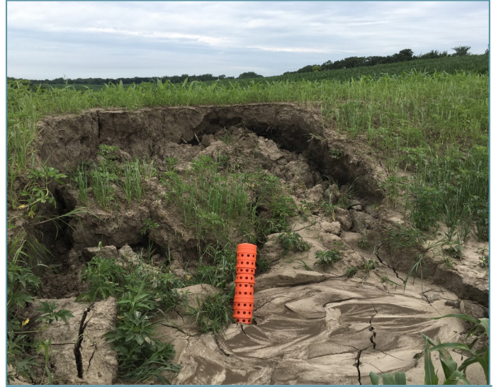
Storms in June 2020 damaged the recently constructed project.
