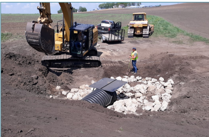
Rock inlet protection and an anti-vortex hood were installed at the upstream end of the pipe.
