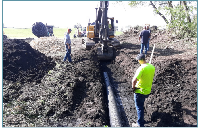
A support tile was installed, offset from the center of the waterway.
