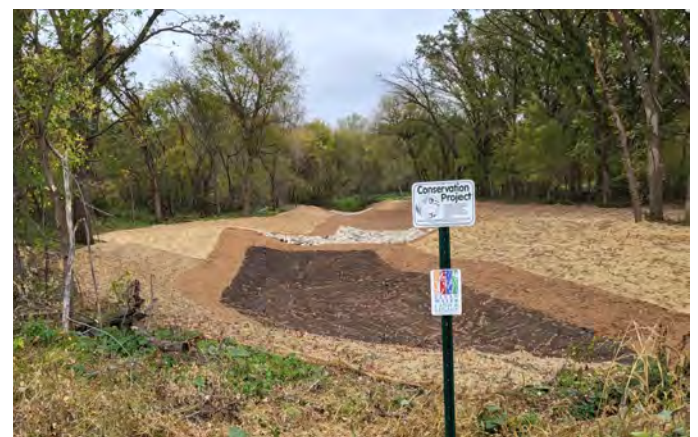
The completed project will capture sediment, reduce future erosion, and protect downstream portions of Trout Brook.
