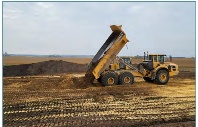
Borrow material was hauled to where it was needed for constructing the berm.
