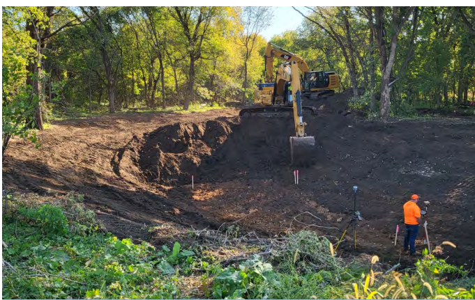
A basin to capture sediment was excavated on the upper end of the project.
