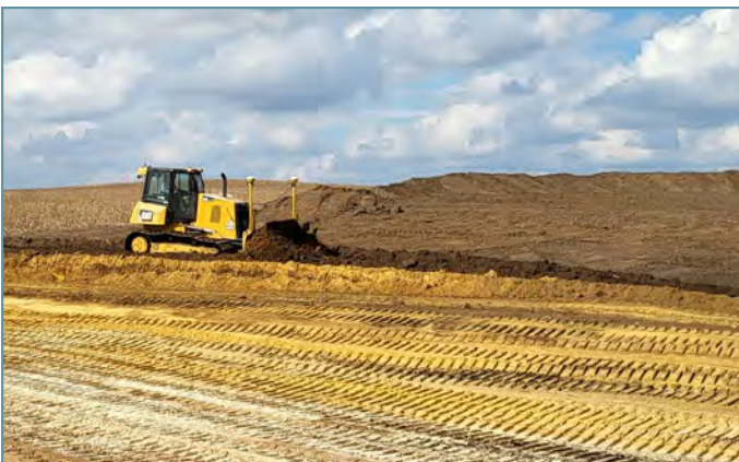
Berms for each basin were constructed to hold back surface water runoff and slowly release the runoff through the underground outlets.
