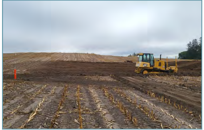
Underground outlets were installed and topsoil was stripped from the construction areas.
