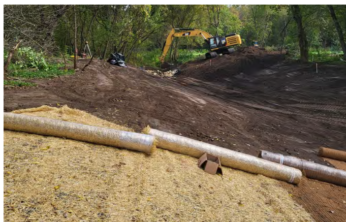
Construction areas were seeded with a perennial seed mixture and stabilized with erosion control blanket.
