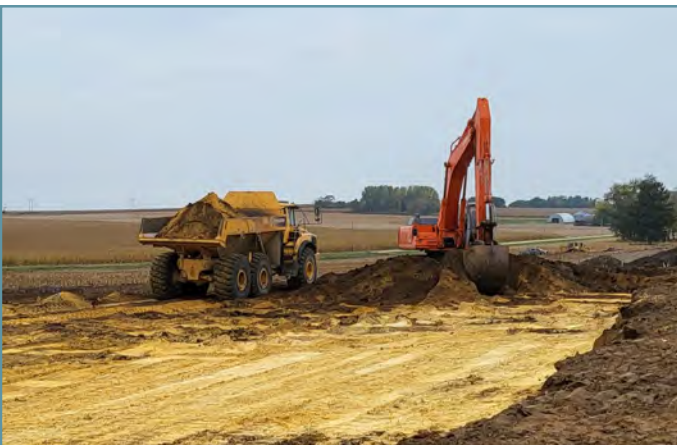
In-field borrow areas were used as sources of material to construct the berm.
