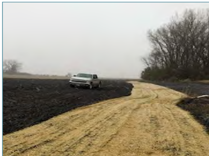
Erosion control blanket was installed in the center of the waterway after seeding.
