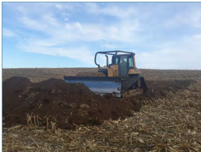
Topsoil was stripped from the project location. The topsoil was replaced after basin grading.
