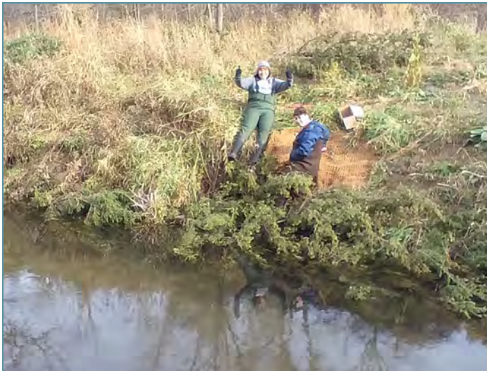
Crews installed cedar tree revetments at Trout Brook in Miesville Ravine Park Reserve to stabilize eroding banks.
