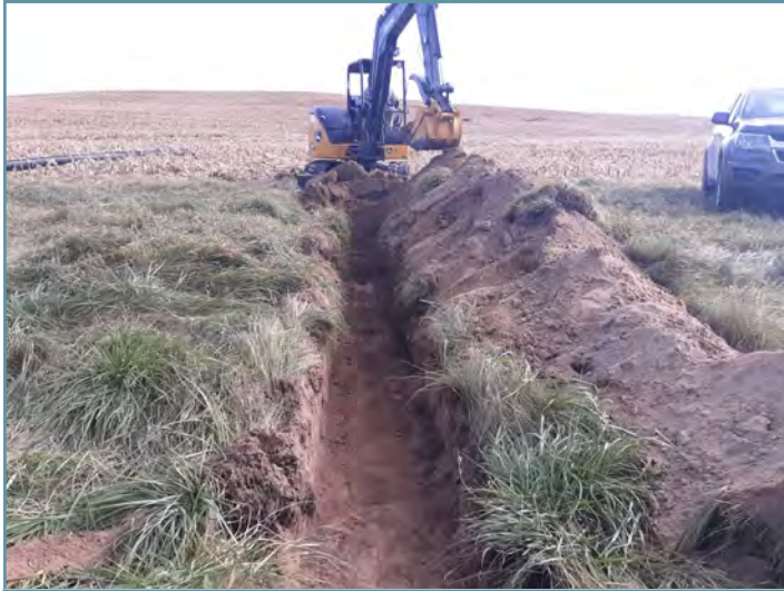
An underground outlet was installed that will discharge to an existing grassed waterway.
