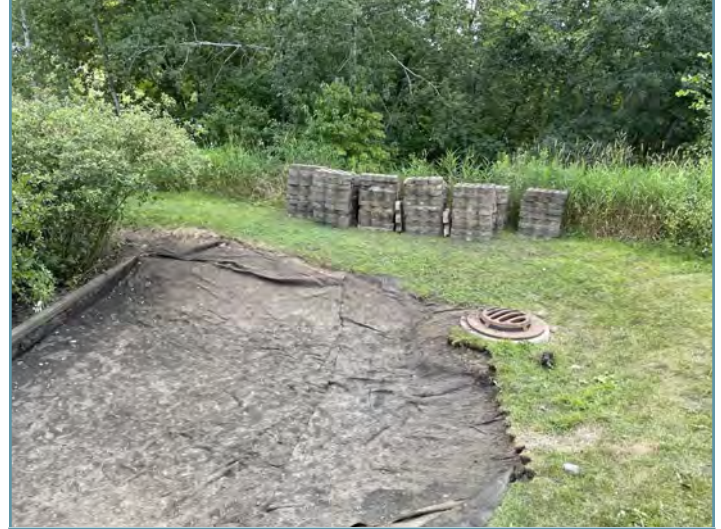
Crews clear accumulated sediment and remove turfstone pavers from a rain garden pre-treatment basin at Jensen Lake.
