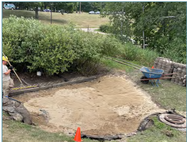
The Jensen Lake pre-treatment basin is graded and leveled before the turfstone pavers are re-installed.
