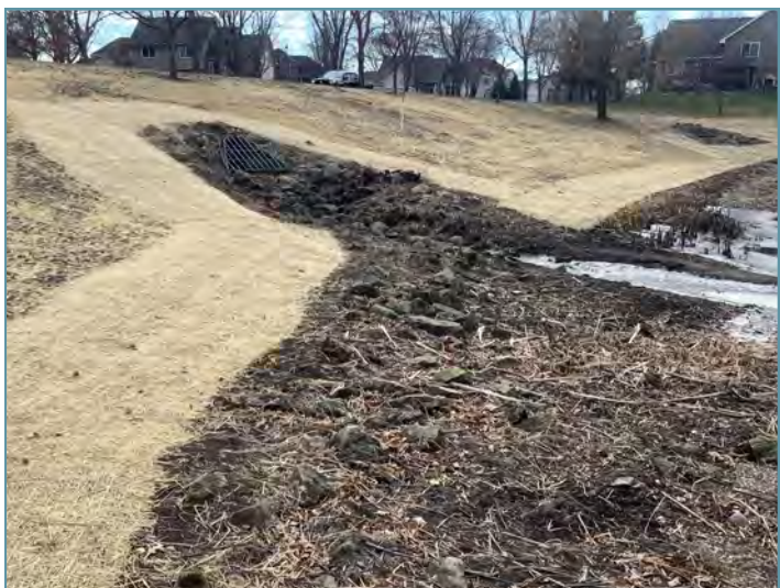
After seeding, natural net erosion control blanket was installed around perimeter of pond.
