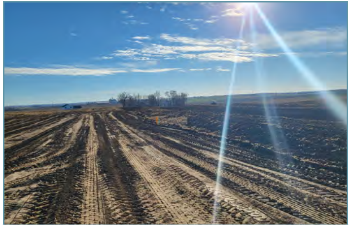
The completed basins will reduce soil loss and reduce future erosion in the field.
