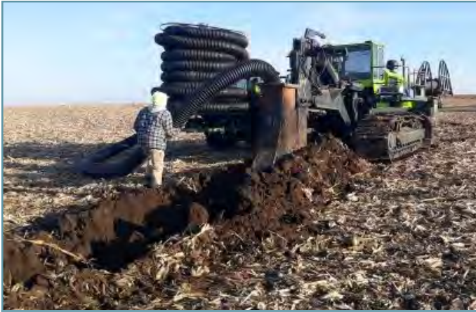
An underground tile outlet was installed which will convey water from the basins to a stable outlet.
