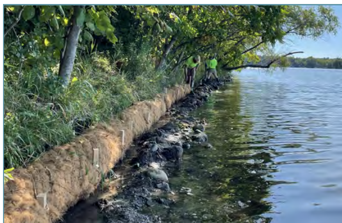
Coir logs were installed along the toe of the slope and the logs were secured with stakes and rope.
