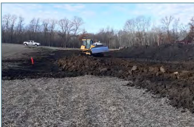
An underground outlet and embankment were constructed to retain surface water runoff at the site of each basin.
