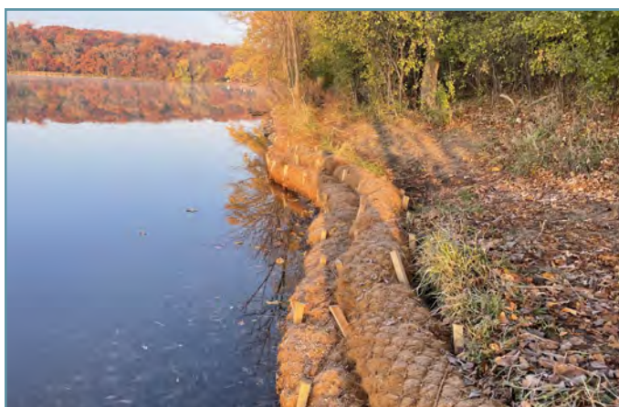
The completed project will reduce future erosion and reduce the amount of sediment that reaches Crystal Lake.
