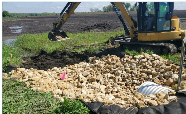
A rock plunge pool was constructed at the top of the eastern waterway to dissipate energy of water from the culvert.
