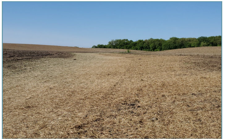
All three waterways had erosion control blanket and mulch installed to reduce erosion until grass is established.
