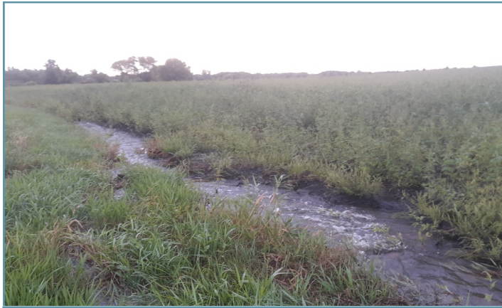
Concentrated water flow was causing erosion in the existing grassed areas.
