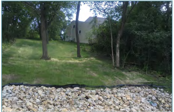
The completed project will minimize erosion on the slope and reduce sediment reaching downstream waterbodies.
