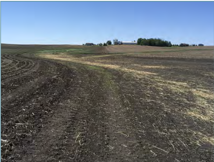
After final grading, the waterway was seeded with a perennial grass mixture.
