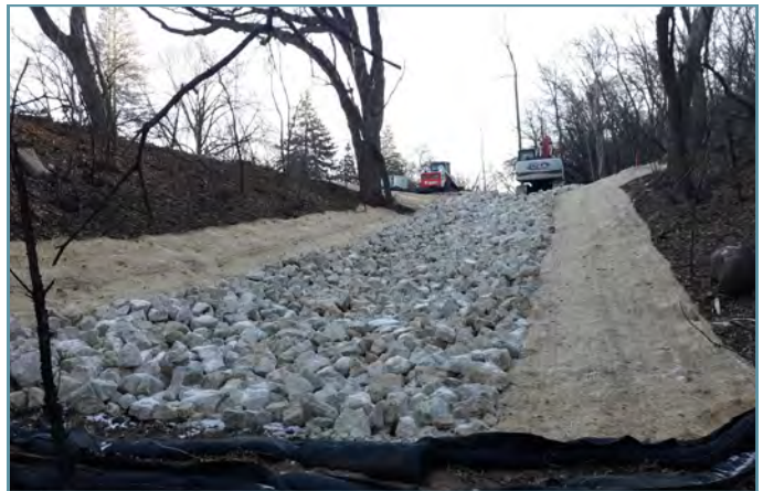
A rock lined channel was constructed to convey runoff down the remainder of the slope.
