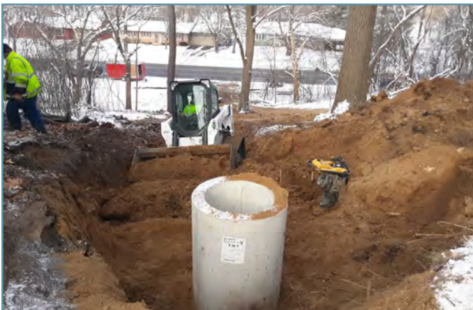
After selective tree clearing, pipes were installed to convey runoff down the steepest part of the slope.
