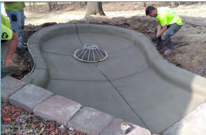
A concrete sump was poured to direct surface water runoff into the pipe and reduce overland flow.
