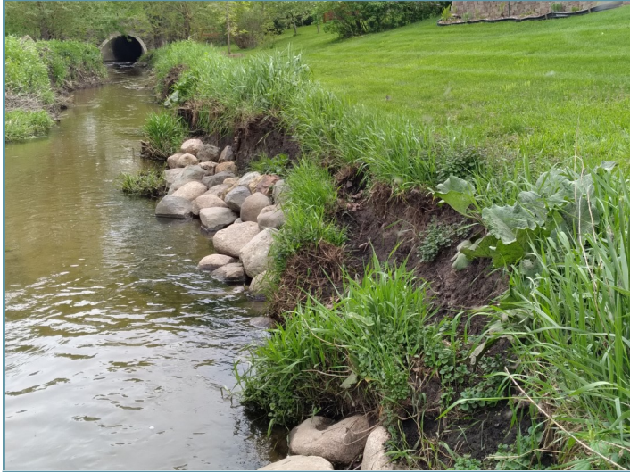
The existing streambank was eroding and lacked deep-rooted vegetation.
