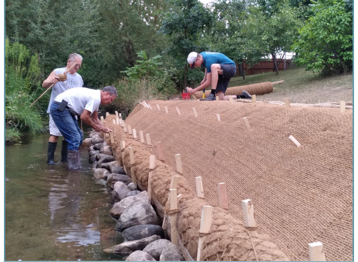
After removal of reed canary grass and turf grass, the project area was seeded with a temporary cover crop and native grasses and wildflowers. Erosion control blanket and coir biogels were installed to reduce erosion.
