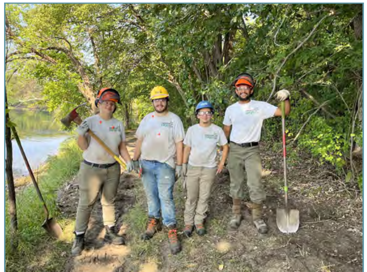
Crews from the Conservation Corps of Minnesota completed the project over the course of two weeks. The project will help reduce future shoreline erosion.
