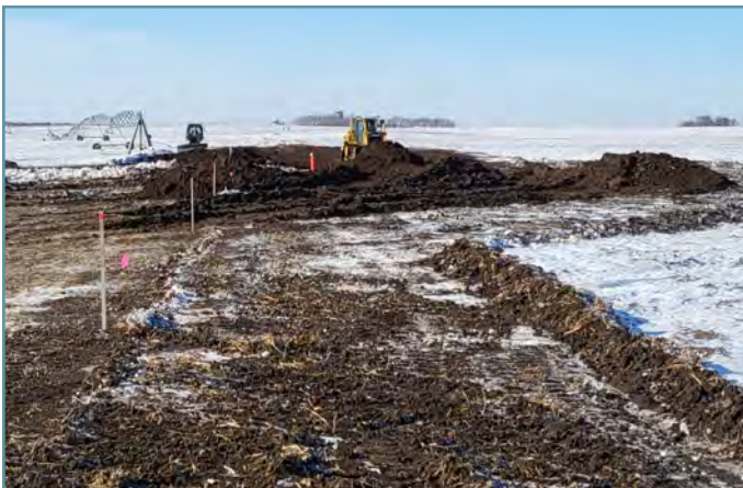
Topsoil was removed and stockpiled, an underground outlet was installed, and the basin and embankment were shaped.
