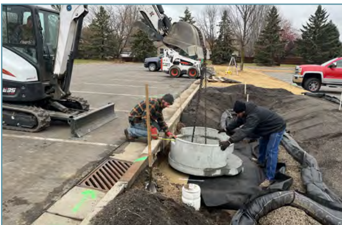
Inlet structures were installed to filter coarse sediment from runoff as it enters the basin.
