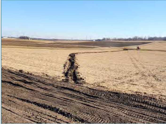
Underground outlets were installed for each basin. The outlets will slowly release water to the downstream channel.
