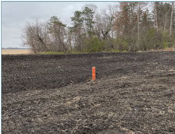
Riser inlets were installed to control the rate of water release from the basin.
