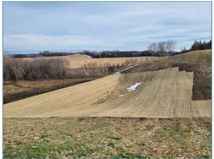
Following embankment construction, the project was seeded and erosion control blanket was installed.
