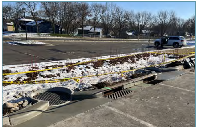
The existing curb was removed and concrete chutes were poured to allow water into the basin.
