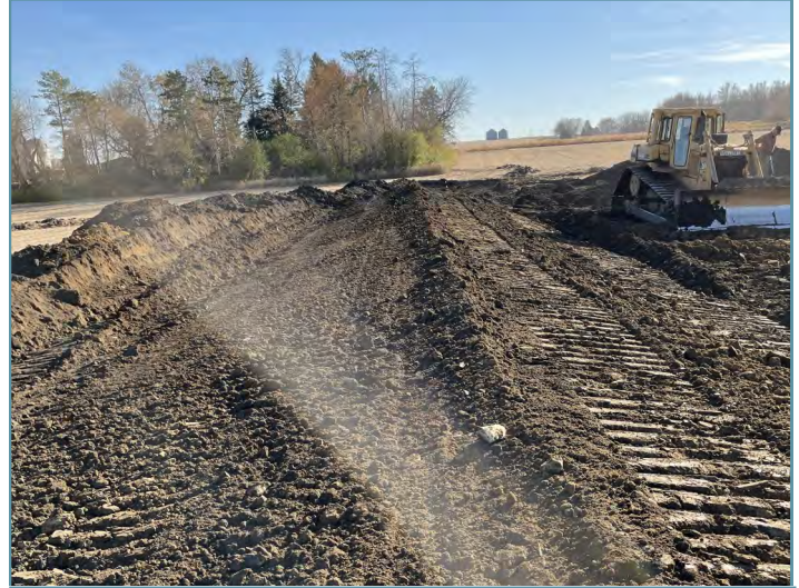
Earthen embankments were constructed to capture and temporarily hold surface water runoff.
