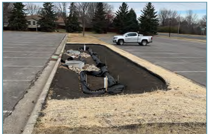
The basin was final graded, side slopes seeded with turf, and prepared for plantings.
