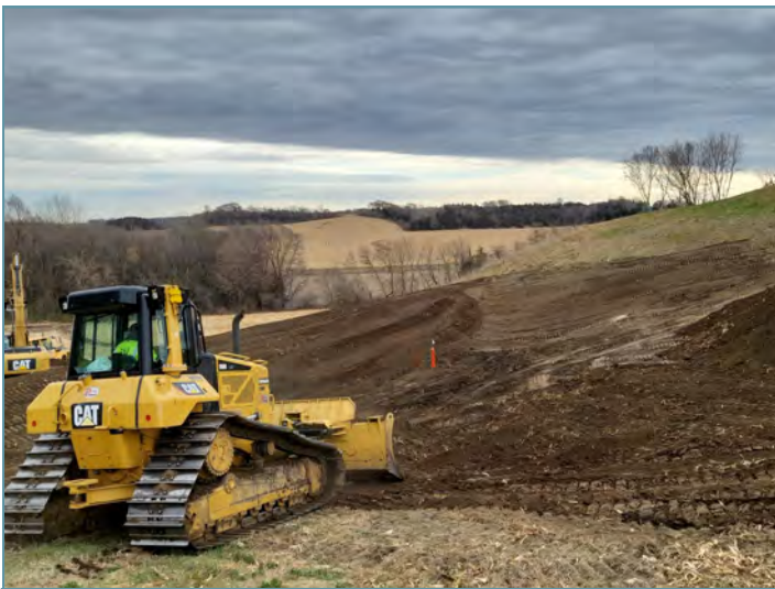
After installation of the underground outlet, an embankment was constructed to capture and temporarily hold runoff.
