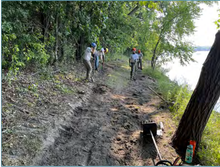
Crews cleared brush and debris from the project area and then hand dug a new trail with shovels and pickaxes which was up and away from the waters edge.
