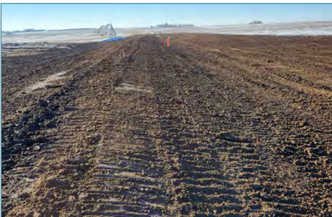
The embankment on the first basin was completed and was then seeded and mulched.
