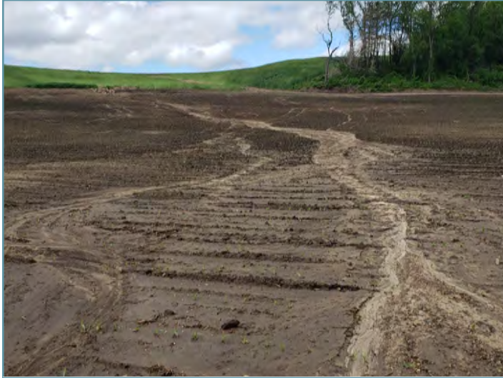
Surface water runoff was causing erosion in the field prior to the start of the project.
