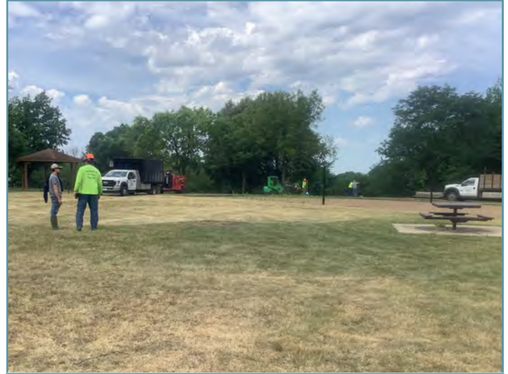
To provide more sunlight for the prairie plants, trees were pruned or removed.
