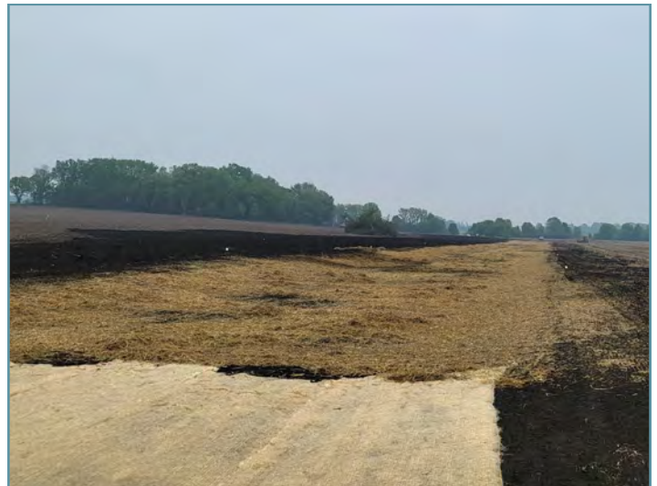
The grassed waterway was seeded with perennial grasses. Mulch and erosion control blanket was used to reduce erosion until vegetation is established.
