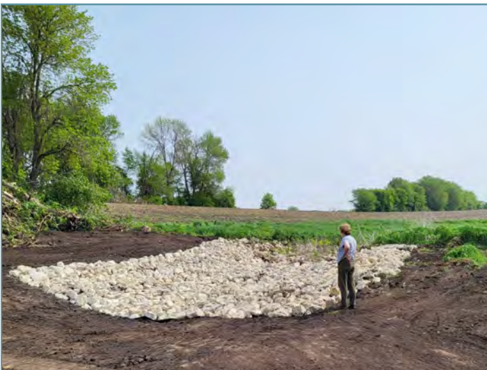
Mary Schwendig (landowner) checking out the progress of the rock lined channel installed at the upstream end of the waterway to collect runoff from adjacent fields.
