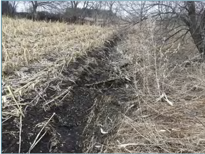
Sediment had filled in the existing grassed waterways. Runoff was flowing outside of the waterways and causing erosion in the field.
