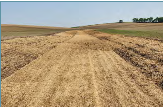
The waterway was seeded, mulched, and an erosion control blanket was installed down the center of the waterway.
