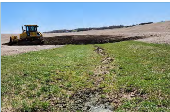
Accumulated sediment in the waterway was removed to improve capacity to convey runoff.
