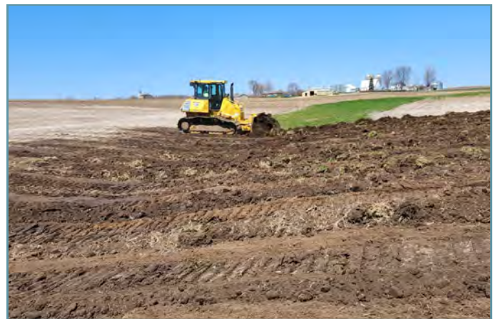
The new waterway was shaped and the removed sediment was dispersed in the field.
