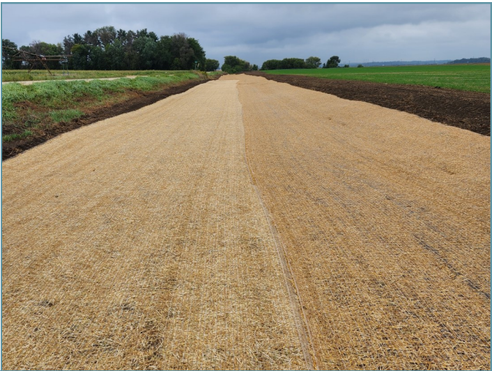
The waterway was seeded with perennial grasses and erosion control blanket was installed down the center of the waterway.
