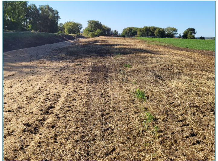
Straw mulch was used for erosion control in areas where erosion blanket was not installed.
