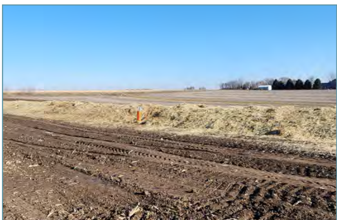
The embankment was seeded. Straw mulch was placed to reduce erosion until vegetation is established.
