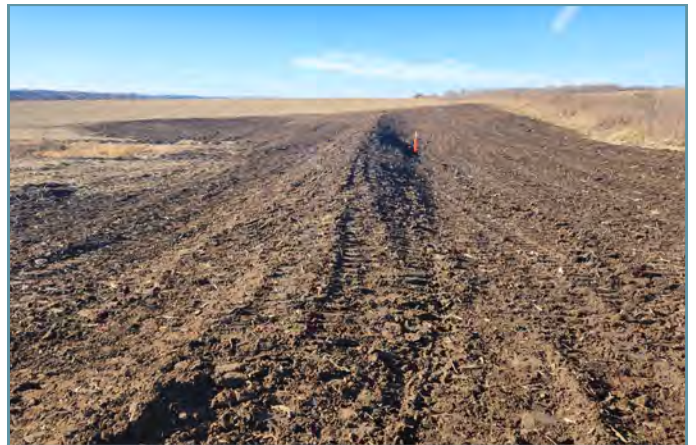
The constructed embankment will capture runoff and release it through the underground outlet.
