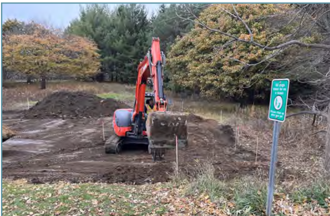
An embankment with a low-flow outlet was constructed to capture and slowly release surface water runoff.
