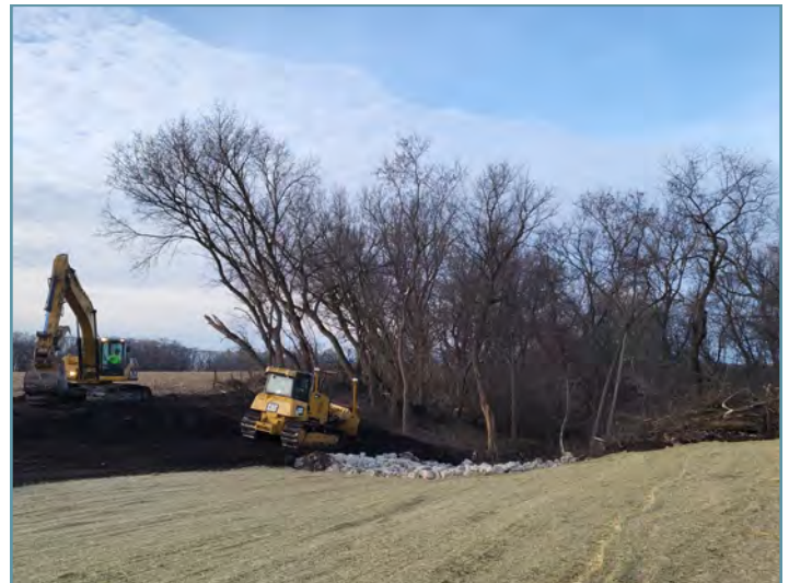
After the site was shaped, topsoil was re-spread and the project area was seeded and covered with erosion control blanket.
