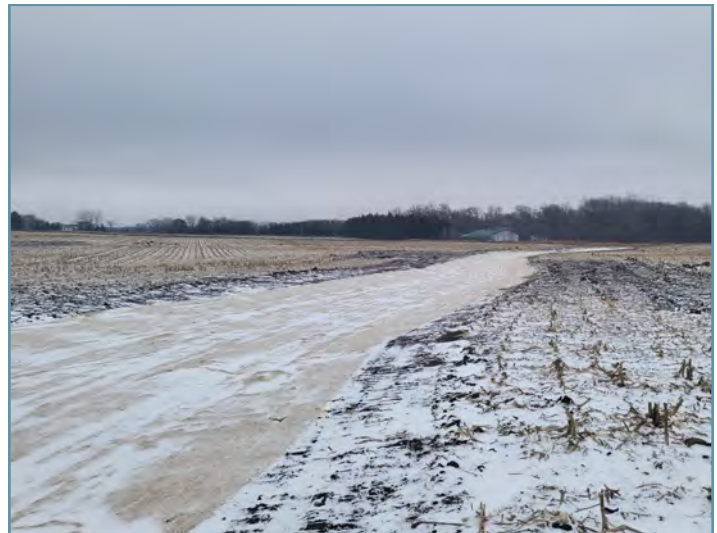
The grassed waterway was dormant winter seeded and erosion control blanket was installed to reduce erosion until permanent vegetation is established.
