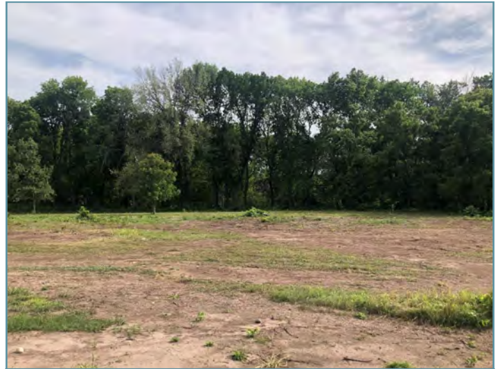
Brush piles were removed and an additional herbicide treatment was used to prepare the site for seeding.
