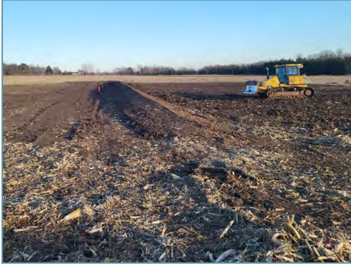
A water and sediment control basin was constructed to capture and slowly reduce runoff. A second water and sediment control basin was also constructed upgradient.
