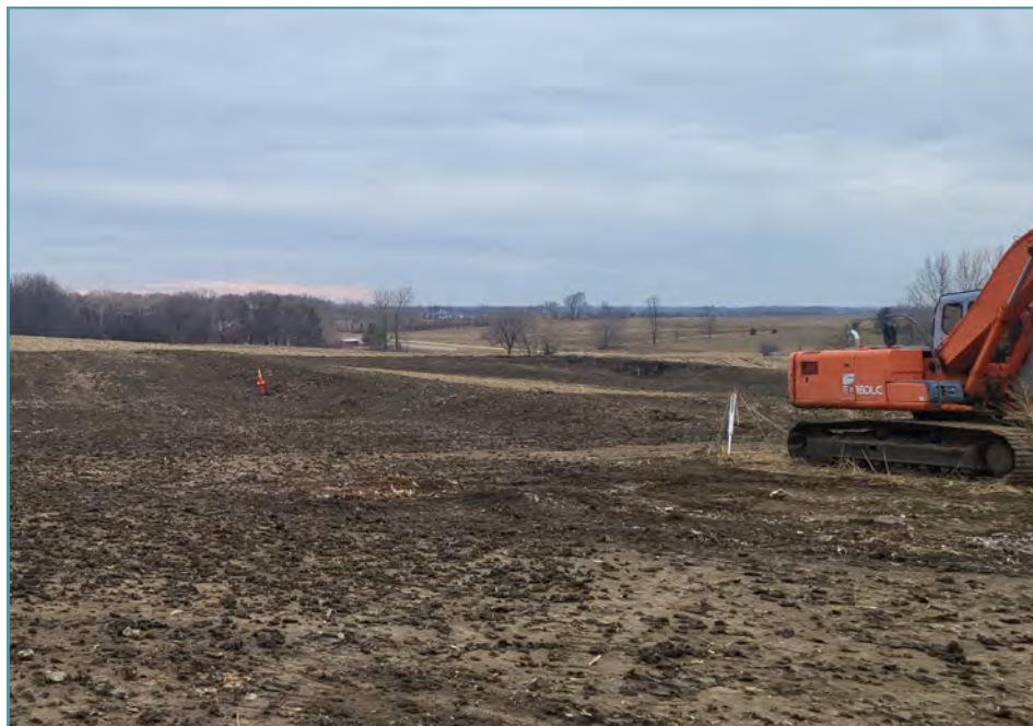
Two water and sediment control basins were installed to capture surface water runoff and slowly release it through underground outlets.
