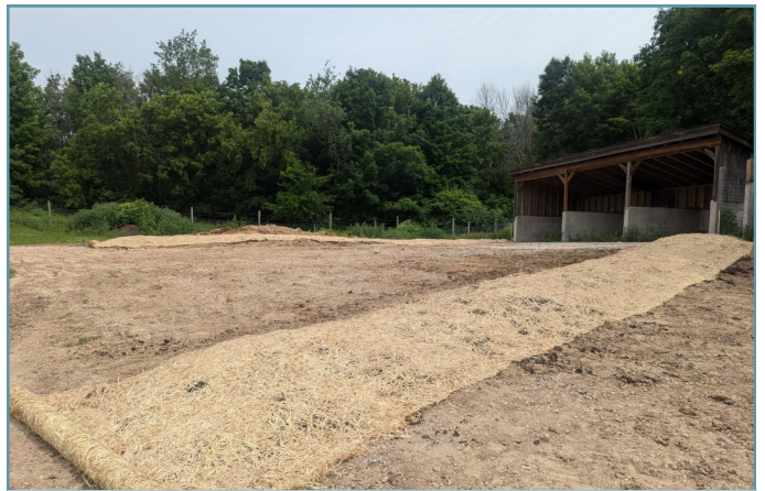
A diversion was constructed to direct any runoff from the pad towards the crop field.
