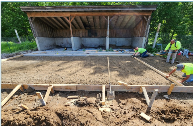
The concrete crew installed and leveled a compacted base in preparation for concrete.
