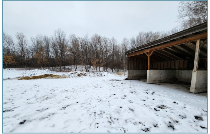
Photo from initial site visit showed unused manure storage due to small area and muddy conditions.
