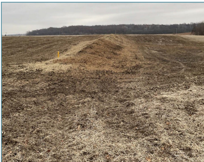
The embankments were seeded with perennial grasses and mulched to reduce erosion until grass is established.
