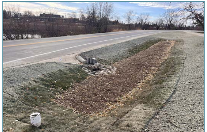
The finished basins will capture, treat, and infiltrate runoff from the road.
