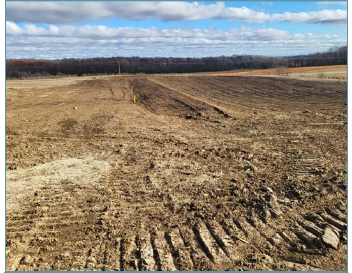
Underground outlets were installed and embankments were constructed in each area to temporarily hold surface water runoff from the field.
