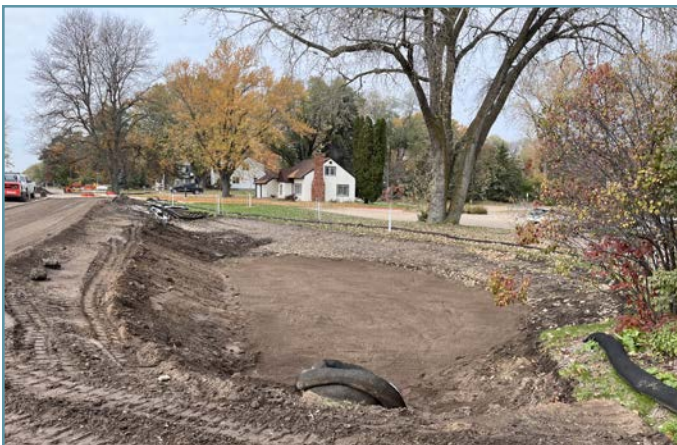
The sand/compost soil mix was placed and ready for final grading around the basins.
