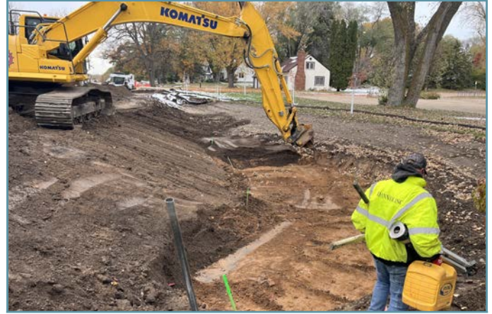
A sand and compost soil mix was added to the basins and the subsoils are "ripped" to promote infiltration.
