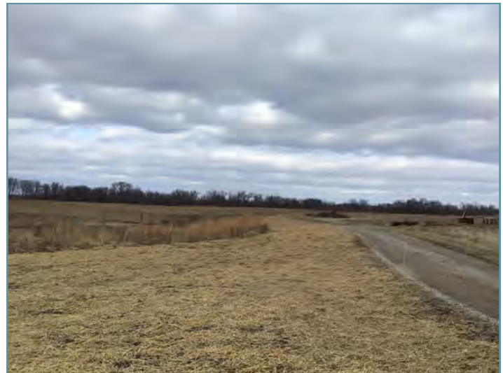
Shortly after seeding, straw mulch was installed in the Wet-Mesic Prairie unit to anchor the seed and reduce the risk of erosion.
